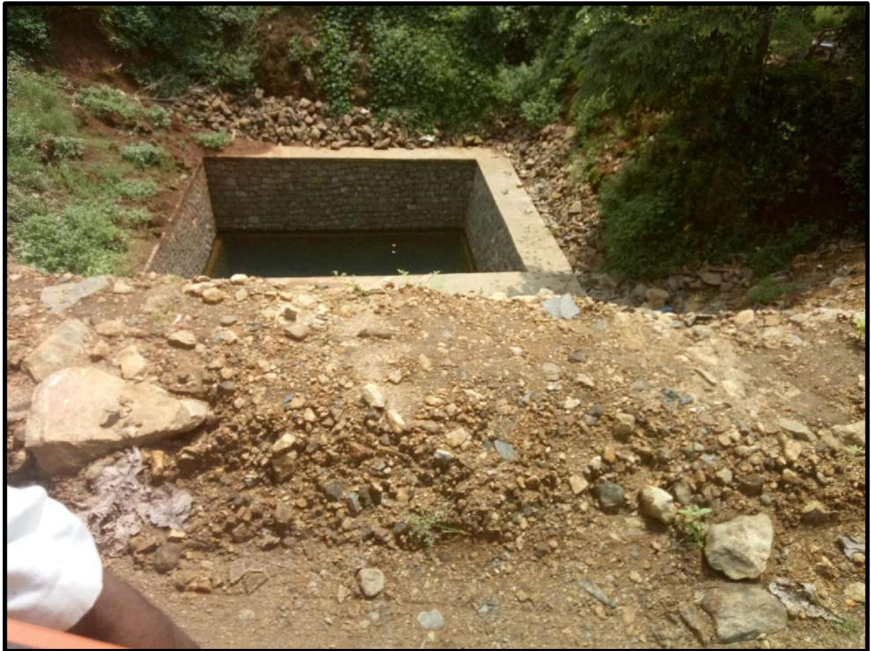
Photograph showing the rain water harvesting tank
